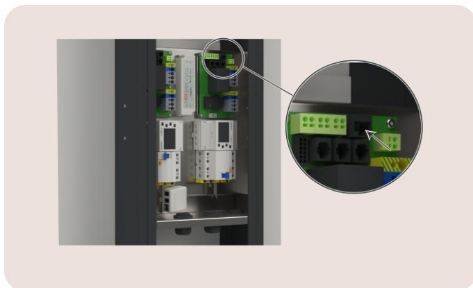
Image 12: View on the A+B port of the relay board
