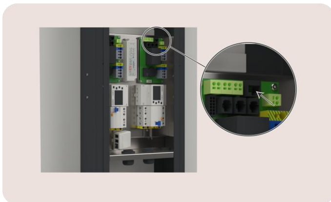
Image 17: View on the A+B port of the relay board
