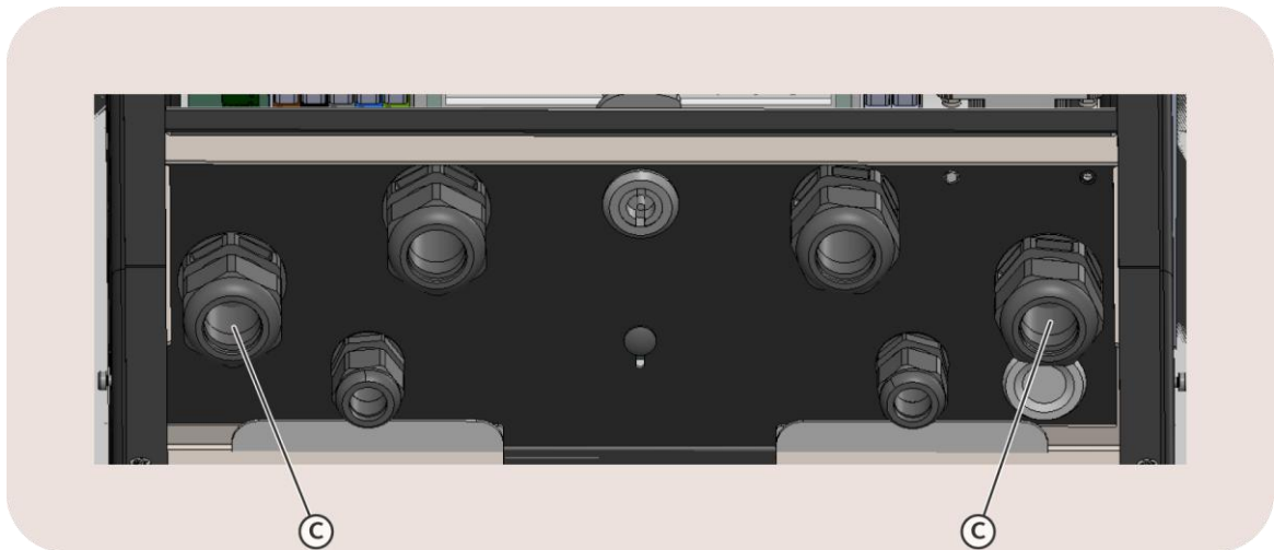
Image 33: View on the cable glands for the charging cables (C).
